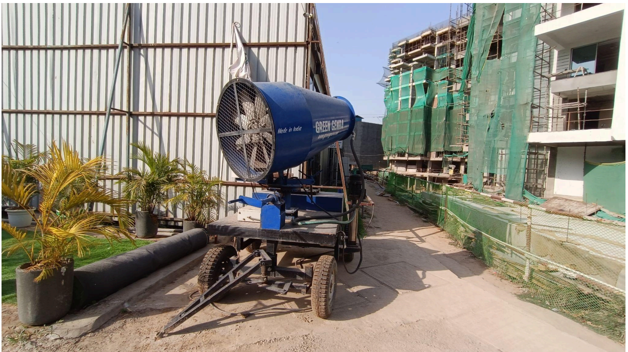
Figure 2. Anti Smog Installed at the Site
